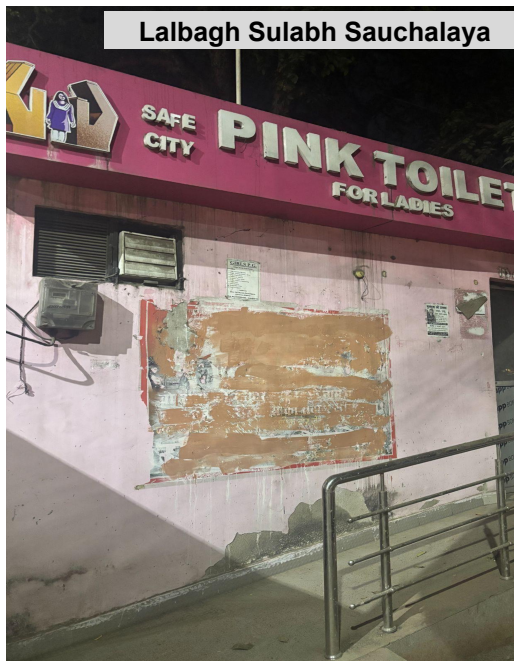
No access to women's toilet
