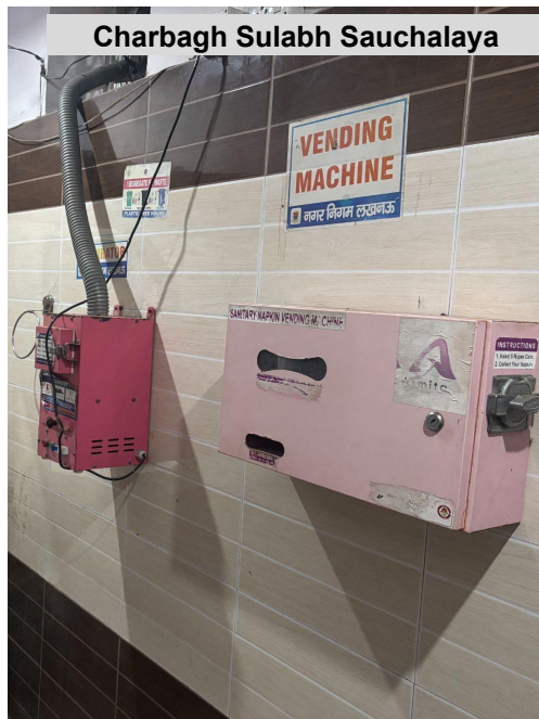
Unkempt sanitary pad dispenser and incinerator
